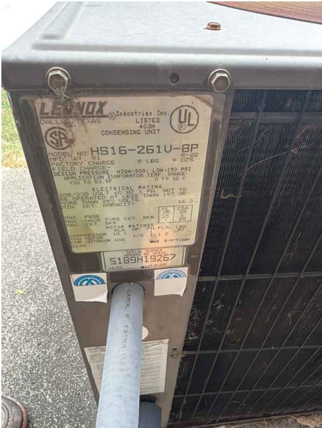
Cooling Outside Unit 3: Brand Lennox Year built 1989
