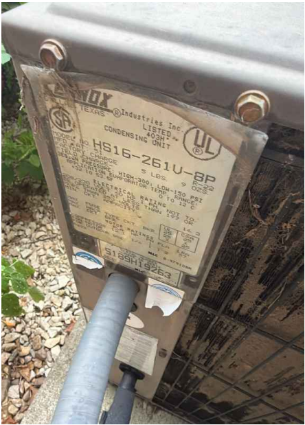
Cooling Outside Unit 2: Brand Lennox Year built 1989
