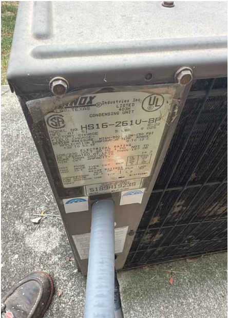
Cooling Outside Unit 3: Energy Source/Type Central Air Conditioner
