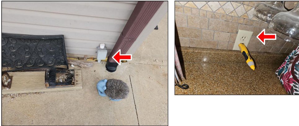
(2) The receptacle on the North side of the home Was not GFCI protected.
